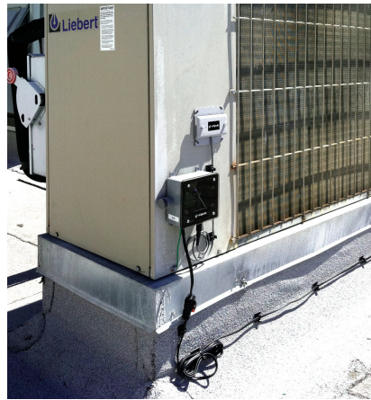
A cellular HVAC monitor on one of Buxton's rooftop air conditioners.
